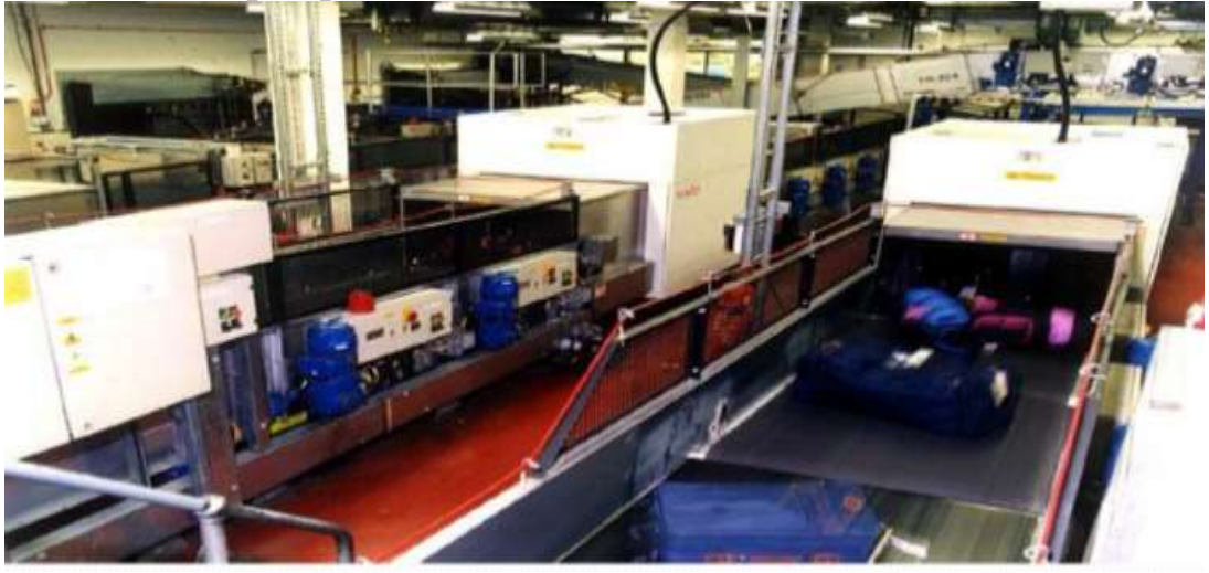
Baggage Inspection Equipment
