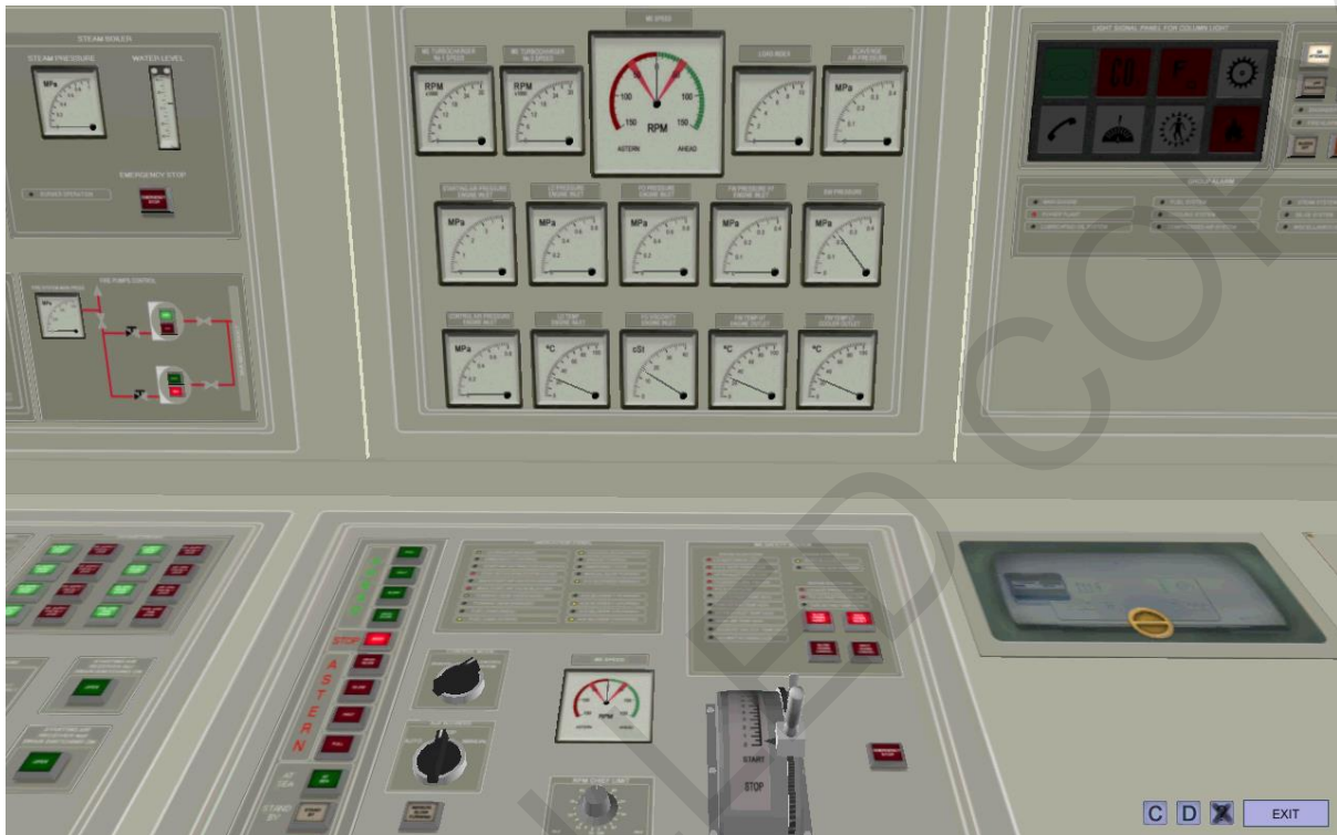
Fig. 9 Engine Room Control Station (ECS)
