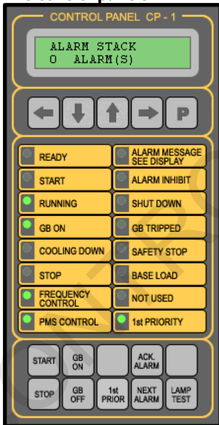
Fig. 95 Control panel - front layout
