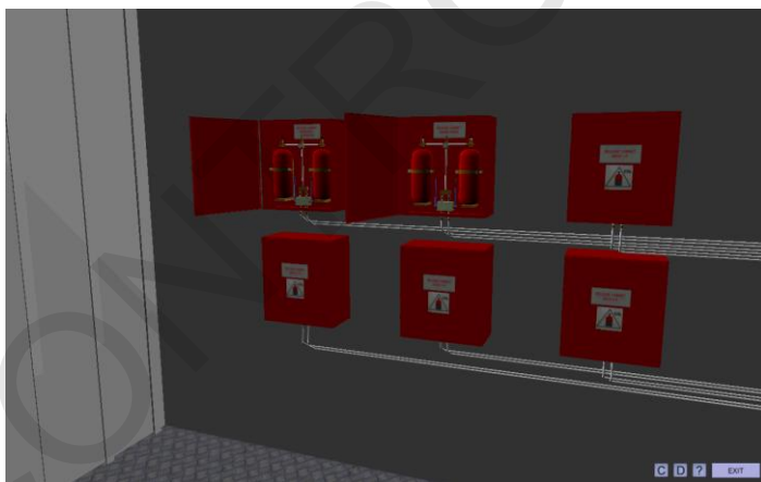
Fig. 88 Control Station (release cabinets)
