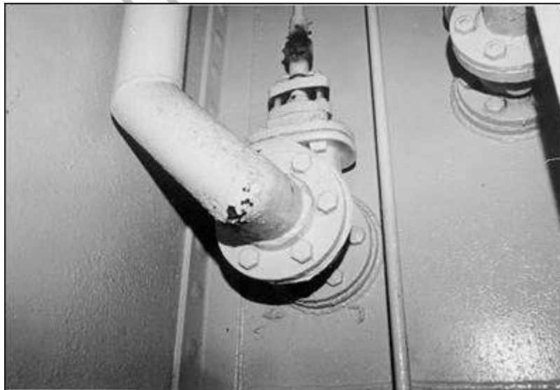
Pipes Passing Through Watertight Bulkhead
